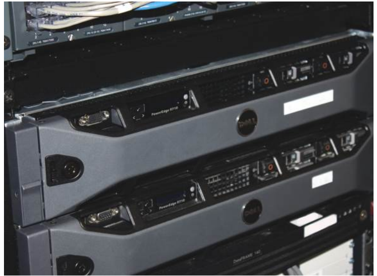
Two of the district's three virtual servers. Each one takes the place of 10 traditional servers.
