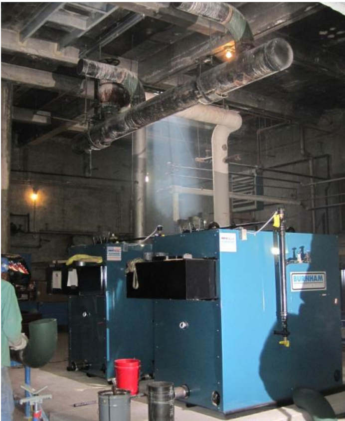
The new boiler at Calumet Park is one of 51 systems replaced at Chicago Park District facilities. In addition to replacing heating and ventilation equipment, the project also included pipe insulation, exterior door and window weatherization as well as remote programmable temperature controls.
